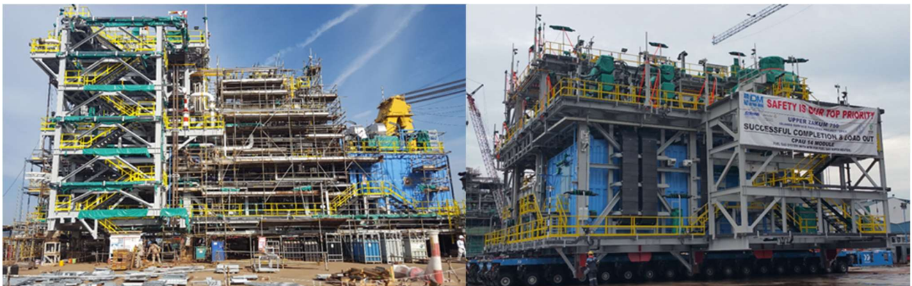
Glycol for Export Gas Compressor
